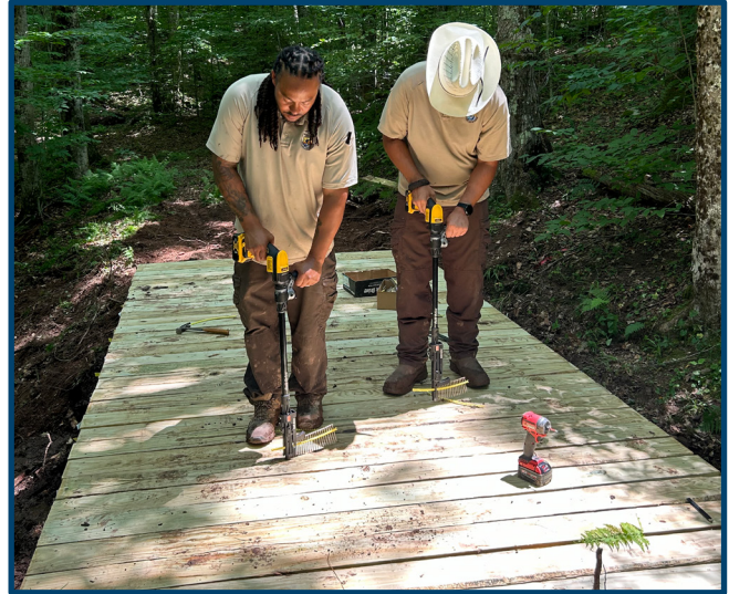
The GAOA team replacing a bridge on a cross-country ski trail by USFWS.
