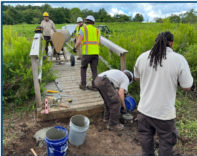
The GAOA team and refuge staff replacing the bridge on South Glade Run trail by USFWS.
